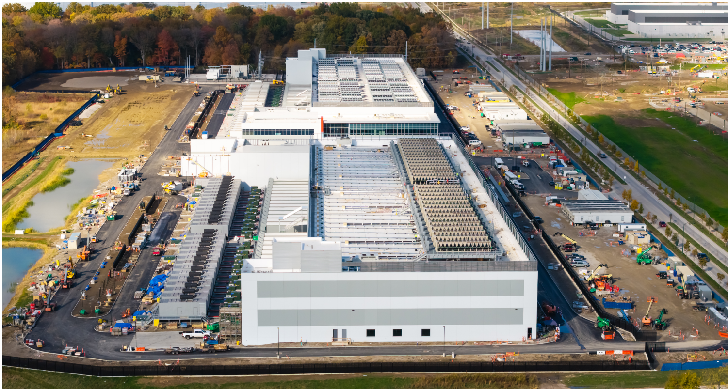
Aerial view of construction of new massive Data center at the suburbs of Columbus, Ohio. As of 2024, the region had 525 data centers — with another 224 planned by 2030
